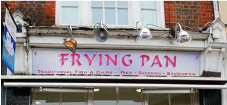
Figure 40 – Unnecessarily extensive lighting.
