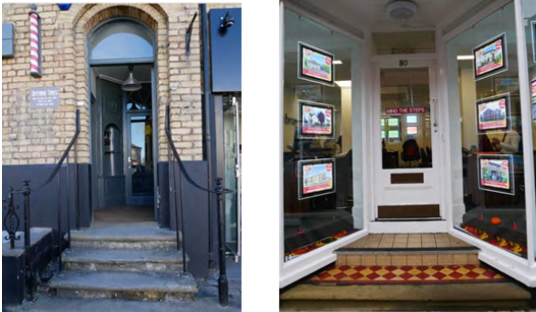
Figure 46 - A historic entrance with original handrails assisting entry (left). An additional step to ease entry (right), however a uniform surface treatment would have been more appropriate.
