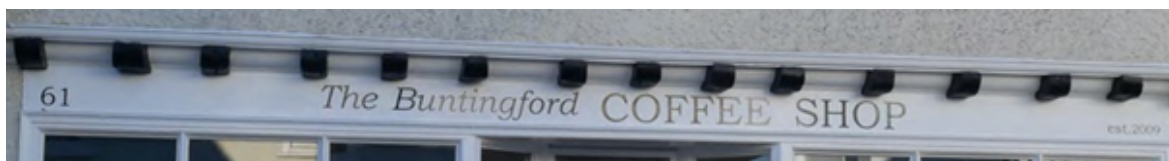
Figure 24 - Various sign and fascia issues
